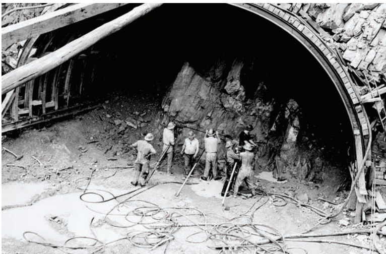
Source 6.23 Displaced persons working on the construction of the Eucumbene–Tumut tunnel, Snowy Mountains Hydro-electricity Scheme [NAA: A11016, 7924]
